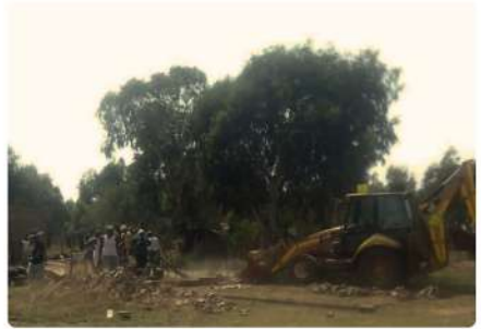
Demolition of the houses/structures reportedly by a mining company called Seriti in KwaMgewana.
