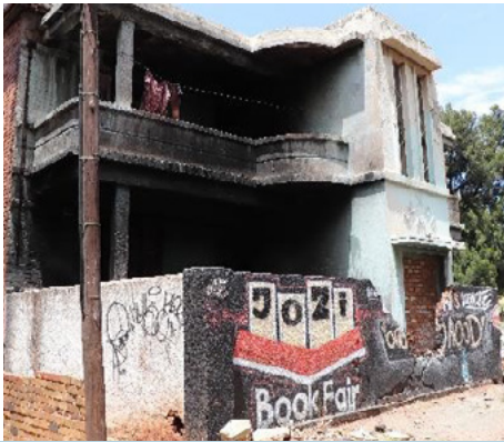
Dilapidated building in the inner city of Johannesburg (Gordon Court and Josana Court)
