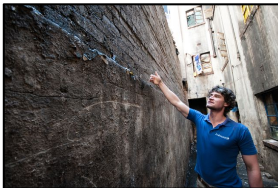
Figure 6: At a surface level we did succeed in our 'quick win' goals. Here, the Planact project officer demonstrates the line up to where the waste used to lie adjacent to the building.
