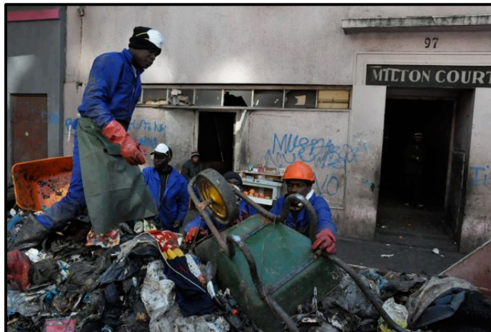
Figure 4: The five men doing the cleaning filled sixteen skips with waste from the building.
